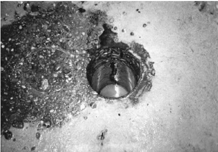
FIGURE 3.42 Hole in pavement after core was drilled at transverse crack in composite pavement.
