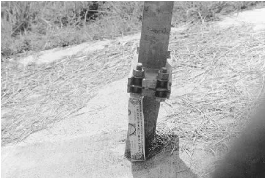
FIGURE 7.52 Improper installation of slip base anchor piece.
