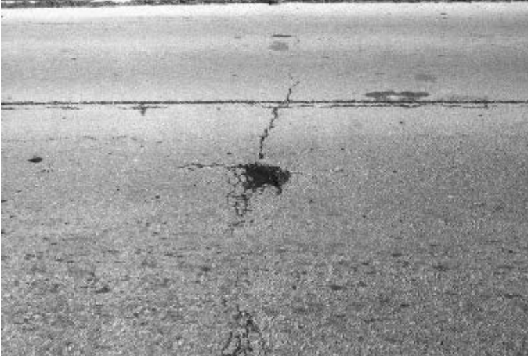
FIGURE 3.33 Example of small pothole in flexible pavement.
