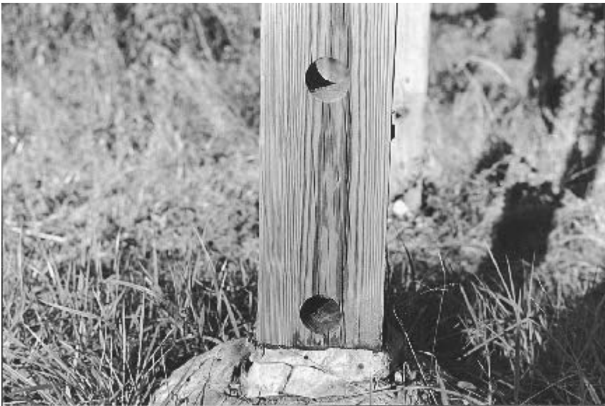
FIGURE 7.62 Weakened wooden post for multiple supports.
