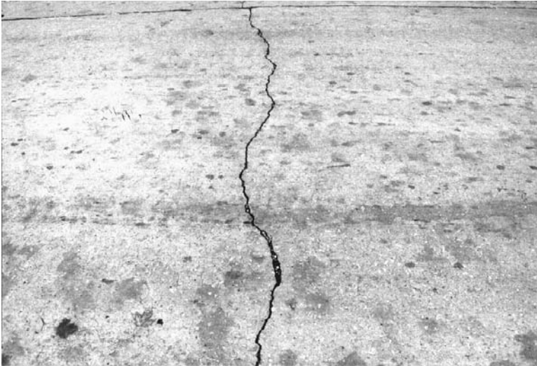
FIGURE 3.26 Example of transverse crack in jointed rigid pavement.
