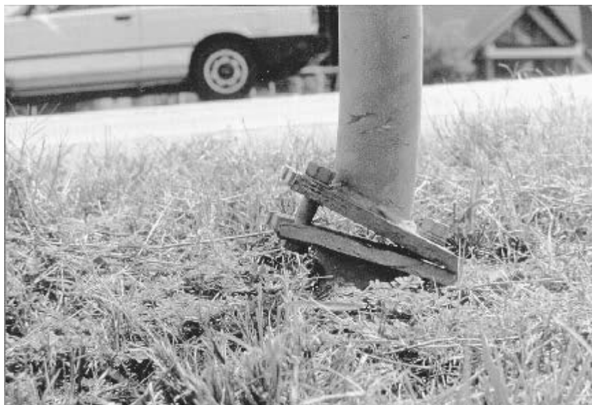
FIGURE 7.26 Loose slip base caused by vibration.
