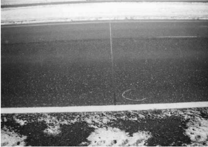
FIGURE 3.8 Joint in composite pavement that has been sawed and sealed.
