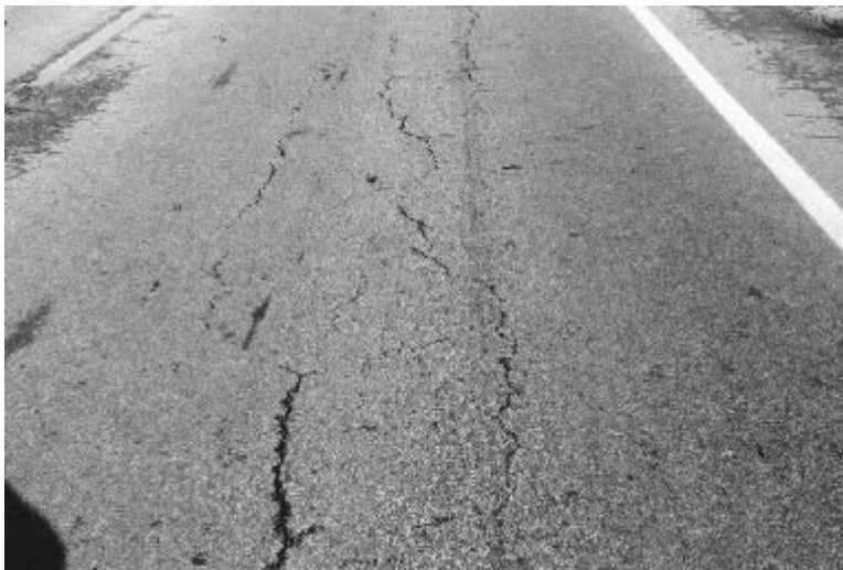
FIGURE 3.36 Example of longitudinal cracking in flexible pavement.
