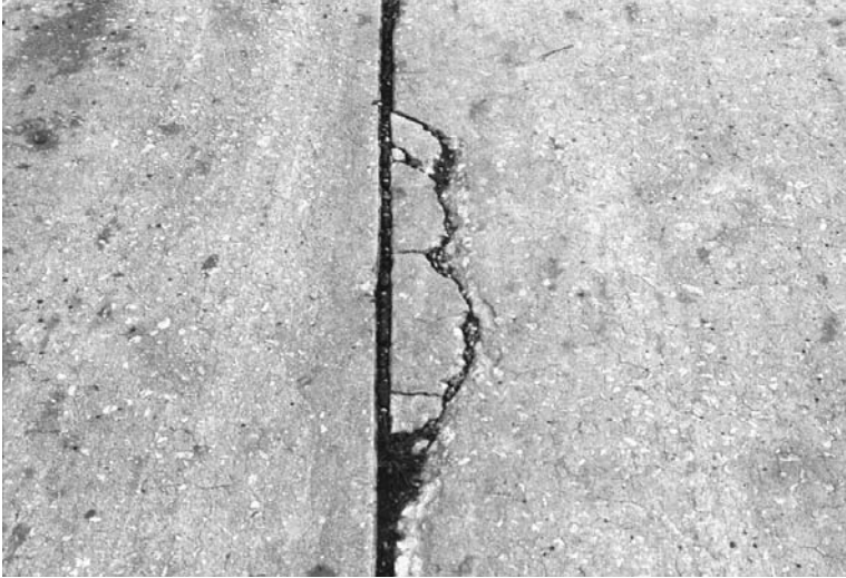
FIGURE 3.25 Example of joint spalling in rigid pavement.
