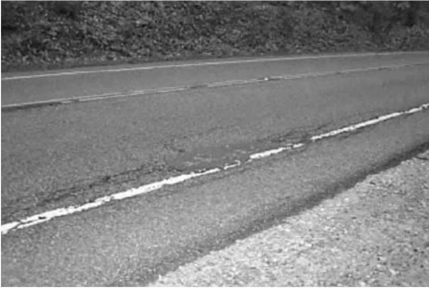
FIGURE 3.57 Localized wheel track and edge cracking.
