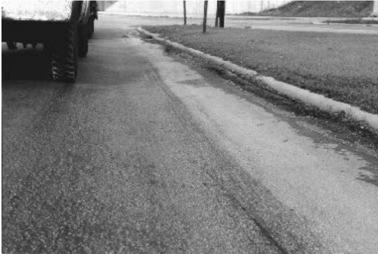
FIGURE 3.35 Example of corrugations in flexible pavement.
