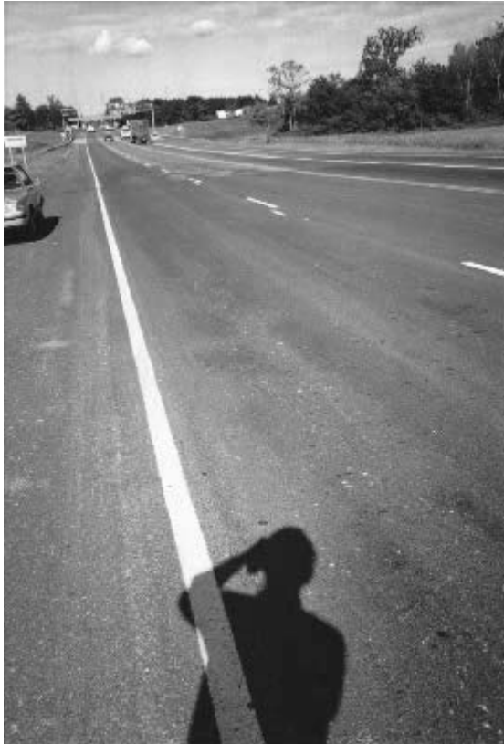
FIGURE 3.32 Example of bleeding in flexible pavement.
