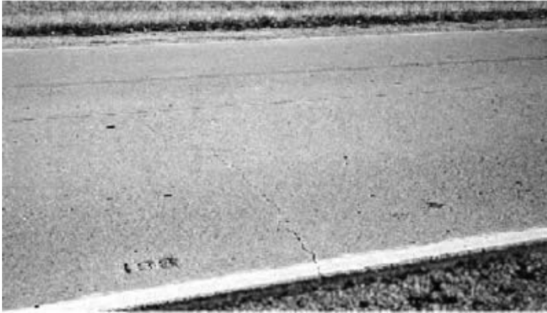
FIGURE 3.55 Hairline crack in rigid pavement.
