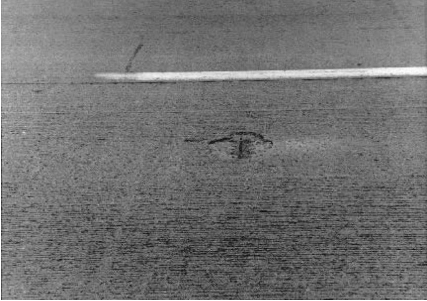
FIGURE 3.23 Example of popout in jointed rigid pavement.
