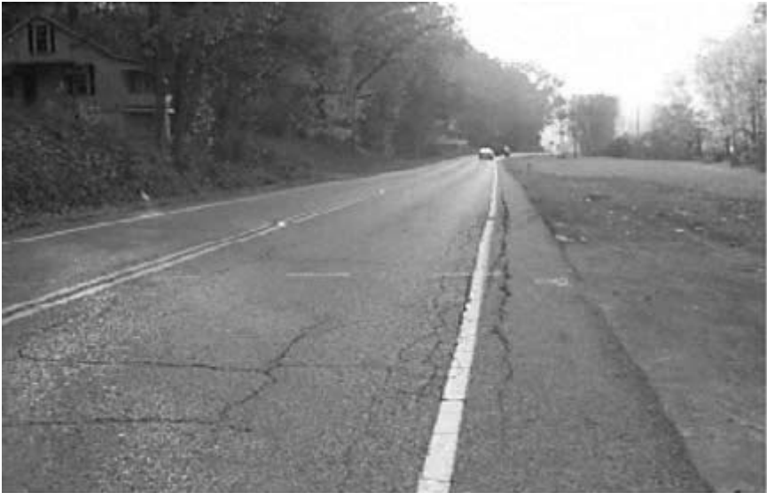
FIGURE 3.58 Localized edge cracking.
