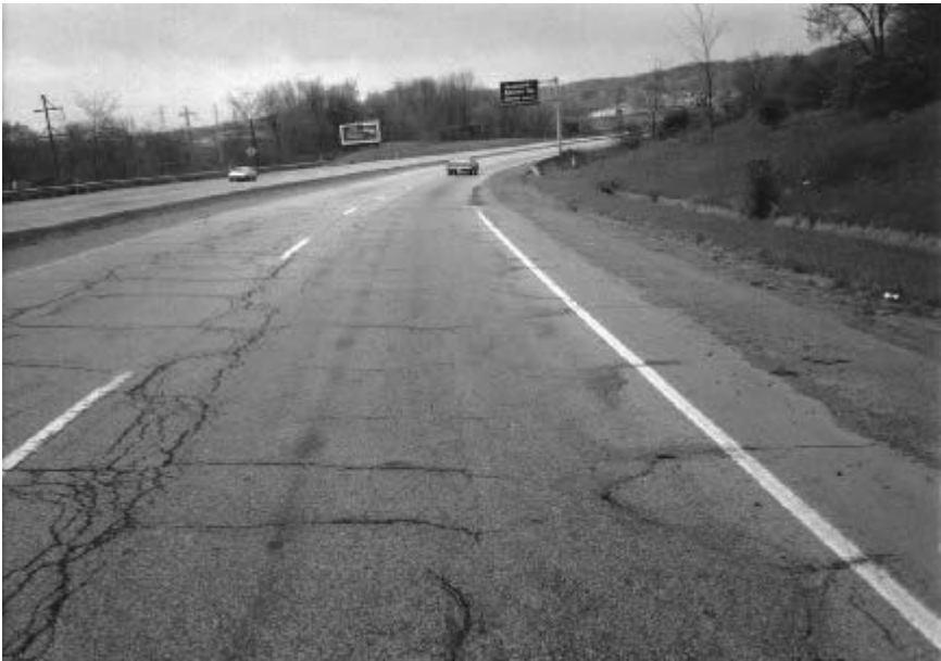
FIGURE 3.38 Example of block cracking in flexible pavement.
