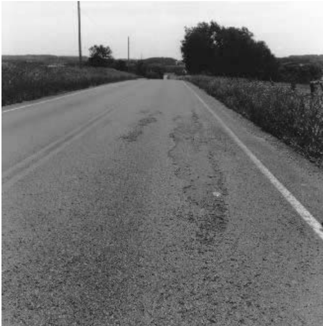
FIGURE 3.31 Example of raveling in flexible pavement.
