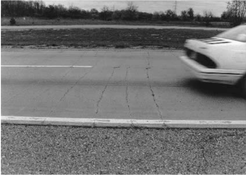
FIGURE 3.29 Example of transverse cracks spaced too closely in continuously reinforced rigid pavement.
