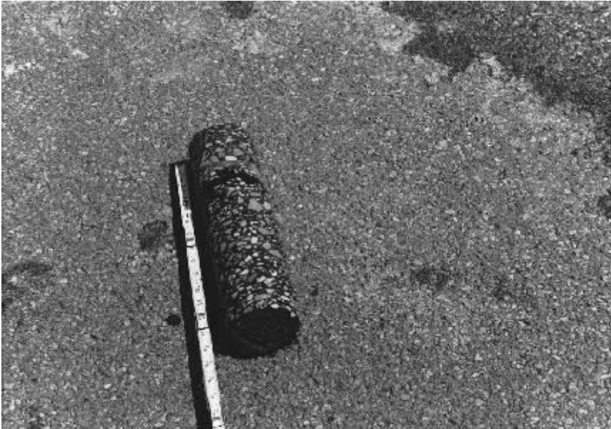
FIGURE 3.45 Core from flexible pavement indicating delamination about 3 in from surface.
