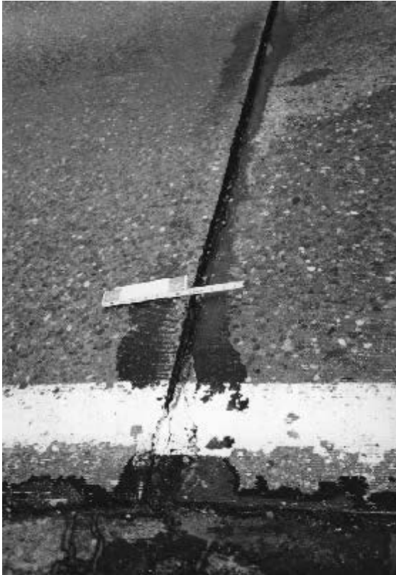
FIGURE 3.24 Example of faulting at joint in rigid pavement; pavement on right is about \frac{1}{2} in lower than that on left.
