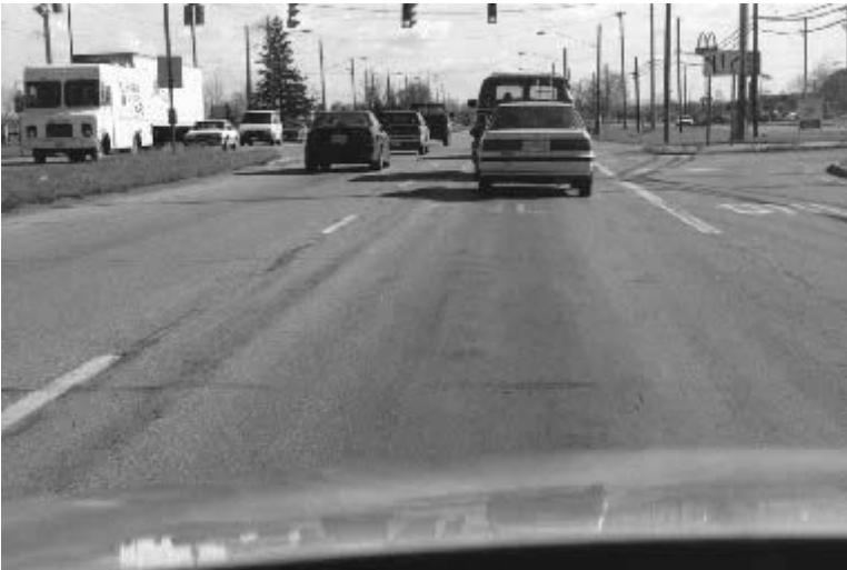
FIGURE 3.34 Example of rutting in flexible pavement.
