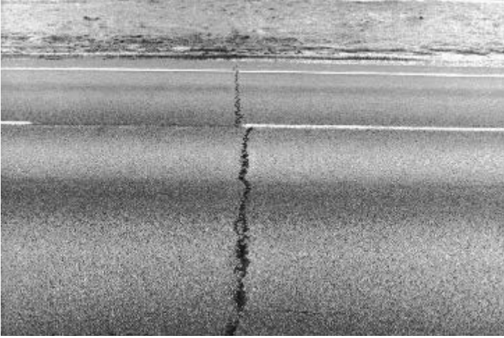
FIGURE 3.37 Example of transverse cracking in flexible pavement.
