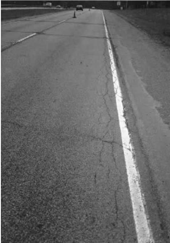
FIGURE 3.40 Example of edge cracking in flexible pavement.
